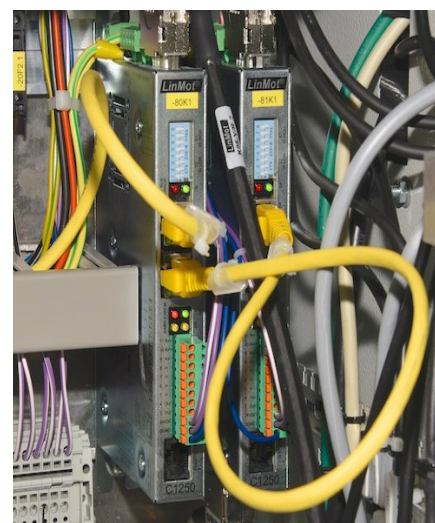
The latest and greatest in the networked age—hidden deep in the electrical enclosure, LinMot axis controllers play a future-oriented role in security and communications to prevent product and brand piracy in the pharmaceutical industry.
